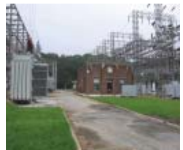
Georgia Power Substation
