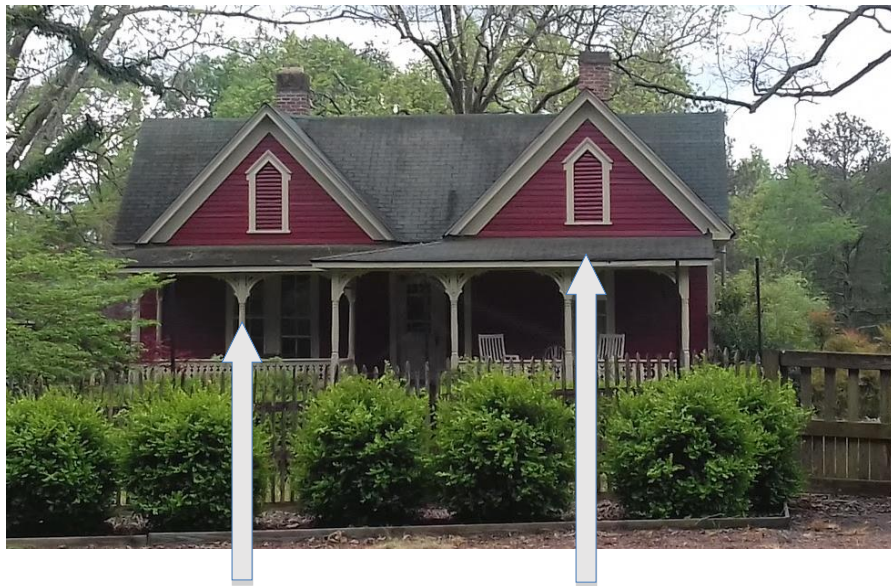
7011 South Goddard Road. Example of decorative porch brackets (left arrow) and decorative vent (right arrow.)
