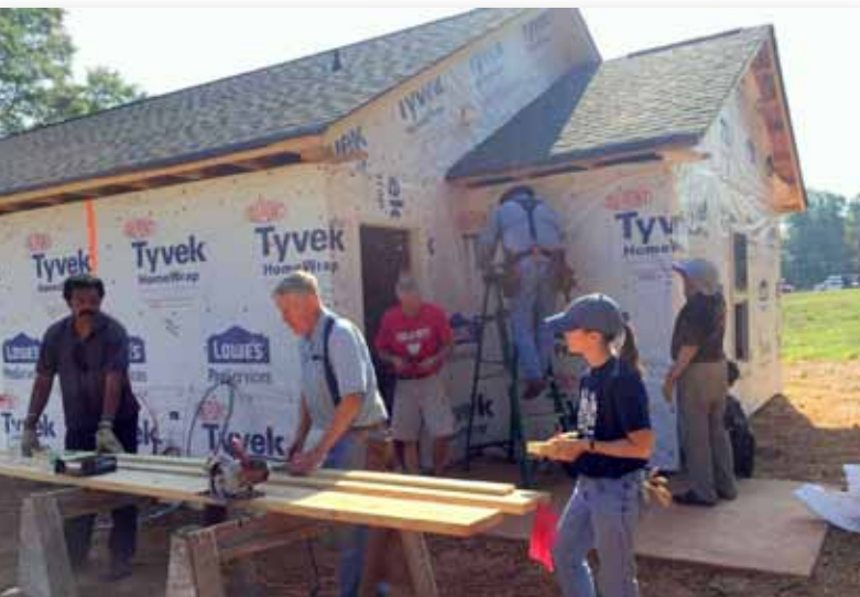
Hiram cuts Hardie Board Siding which volunteers carry to the installation team.
