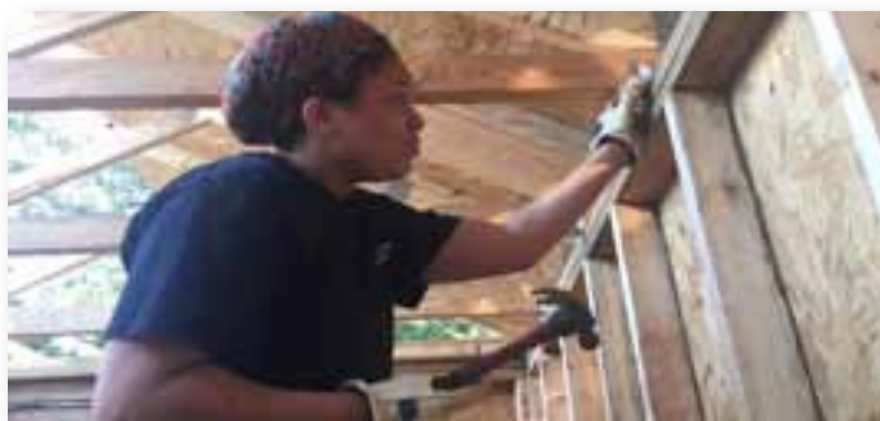
New homeowner Tori Hitchcock and her father were at the build every week!
