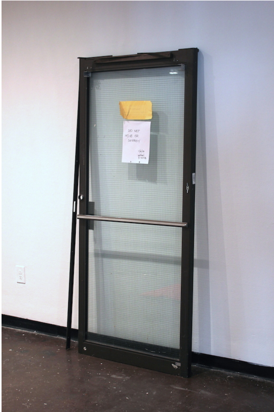
Figure 25 – leaning office door
